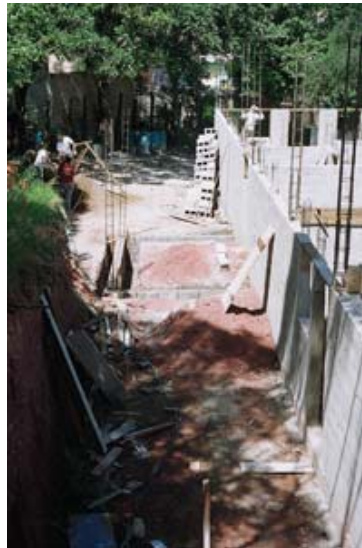
A two-story, concrete block dormitory under construction by local workers at El Hogar, with assistance from work team visitors from St. Peter's Church Weston who mix and load concrete in the rear left corner.
