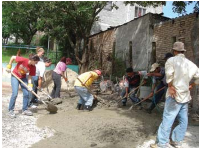
Work team members from St. Peter's Church Weston mix concrete with local workers in Tegucigalpa, Honduras where they spent a week helping to build a new dormitory at El Hogar, a residential school for homeless boys and girls.
